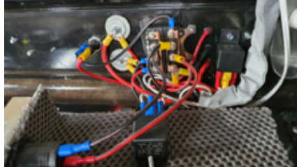
UNCOVERED - Switch, wiring and relays
