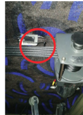
Location of Limit Switch near the winch motor
